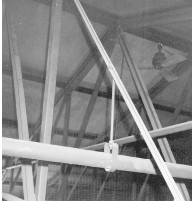
FIGURE 10.15 This is not a good way of supporting collateral load. The pipe should have been hung from a truss panel point.
